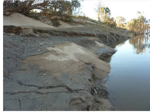
Flood deposition and erosion
